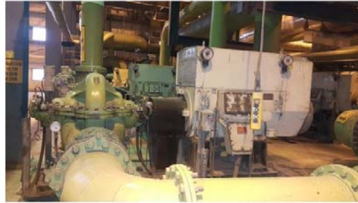
Figure 4: This condensate cooling-water pump experienced chronic cavitation and vibration events that resulted in bearing failures and unscheduled downtime of the Nabha power facility.
