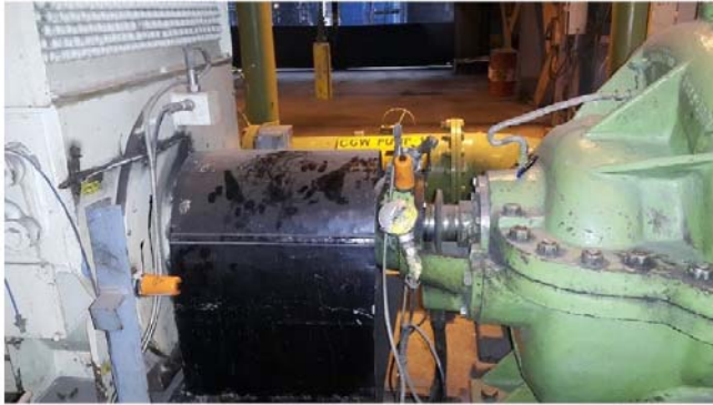
Figure 5: Using past maintenance work orders, plant engineers selected optimum locations to install advanced acoustic-vibration sensors. Courtesy: Nanoprecise Sci Corp.
