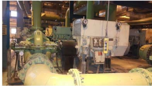
Figure 6: The advanced wireless acoustic sensors were installed using a strong magnet and a two-part epoxy to endure the rigors of this pump's operations. Courtesy: Nanoprecise Sci Corp.
